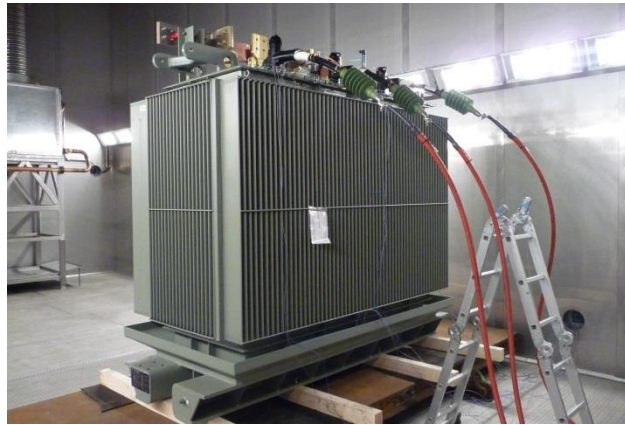
Figure 8: 5.56 MVA Bio-SLIM transformer inside the climate chamber at -30°C
